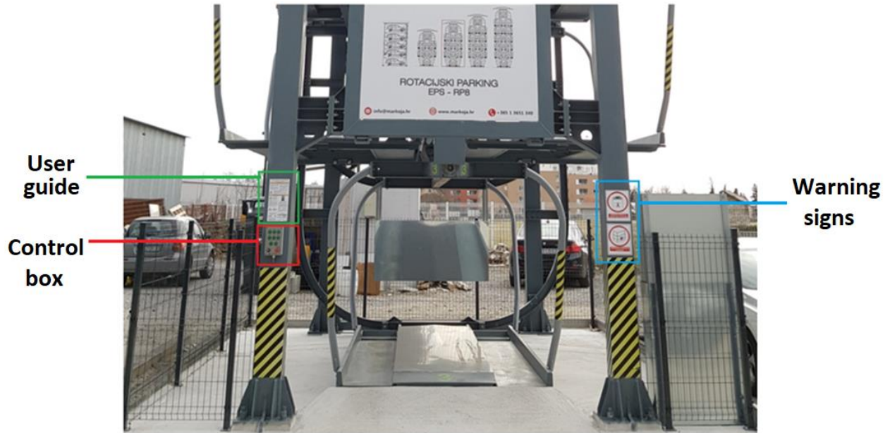
Figure 1: Operation manual and warning signs on the access side of the rotating parking system
