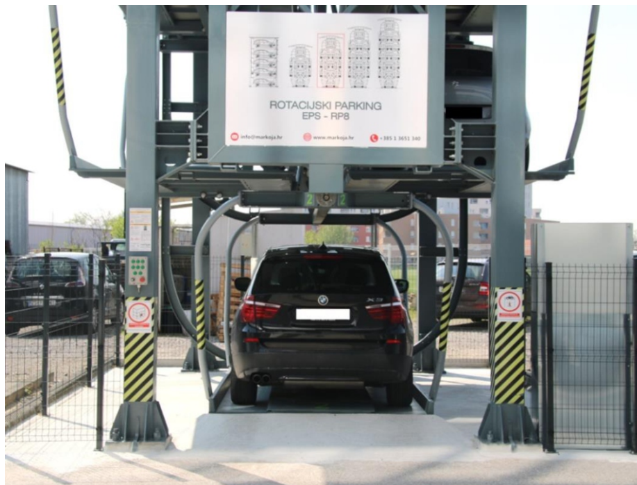
Figure 10: Occupied parking platform at level "0"
